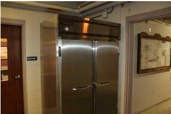
#65 COMMERCIAL KITCHEN, REFRIGERATOR, 2-DOOR REACH-IN
