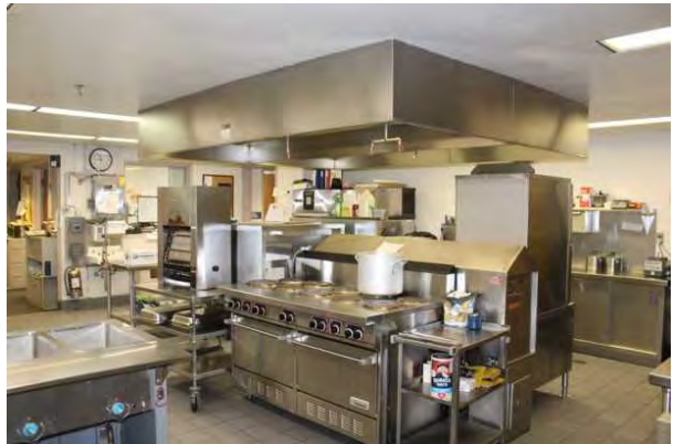
#64 COMMERCIAL KITCHEN, EXHAUST HOOD
