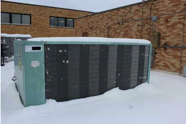
#43 CONDENSING UNIT, SPLIT SYSTEM
