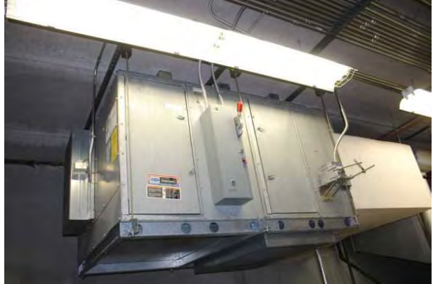
#44 AIR HANDLER (AHU)
