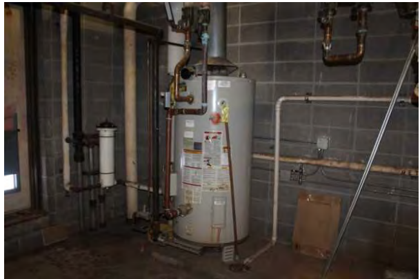
#34 WATER HEATER, GAS
