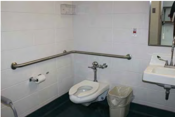
#27 TOILET, COMMERCIAL WATER CLOSET
