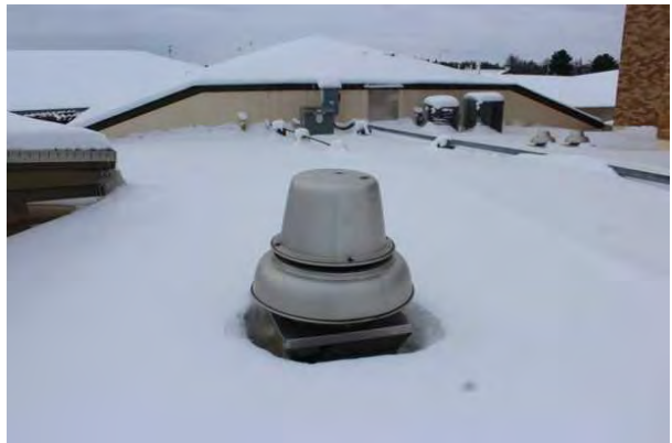
#48 EXHAUST FAN, ROOF
