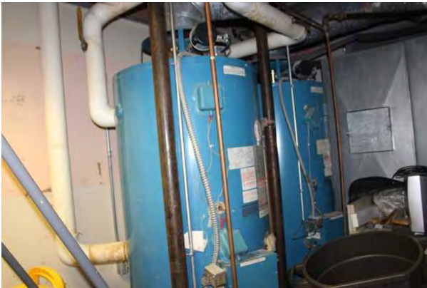
#33 WATER HEATER, GAS
