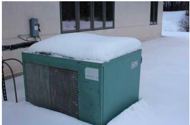
#42 CONDENSING UNIT, SPLIT SYSTEM
