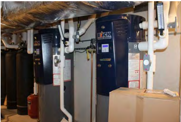
#35 WATER HEATER, GAS
