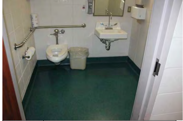
#26 TOILET, COMMERCIAL WATER CLOSET
