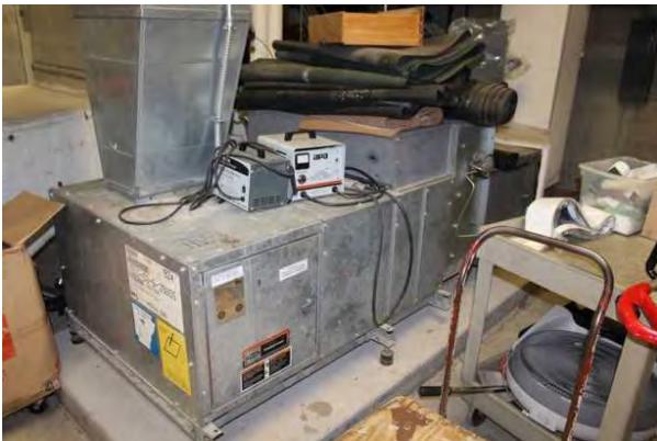
#47 AIR HANDLER (AHU)
