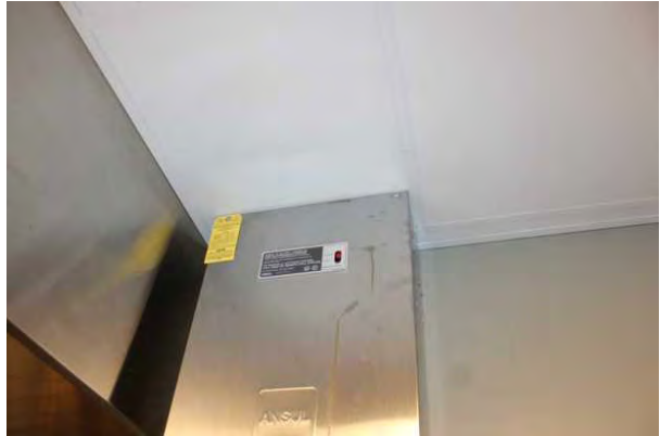
#52 FIRE SUPPRESSION SYSTEM, COMMERCIAL KITCHEN
