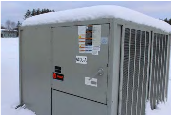
#41 CONDENSING UNIT, SPLIT SYSTEM
