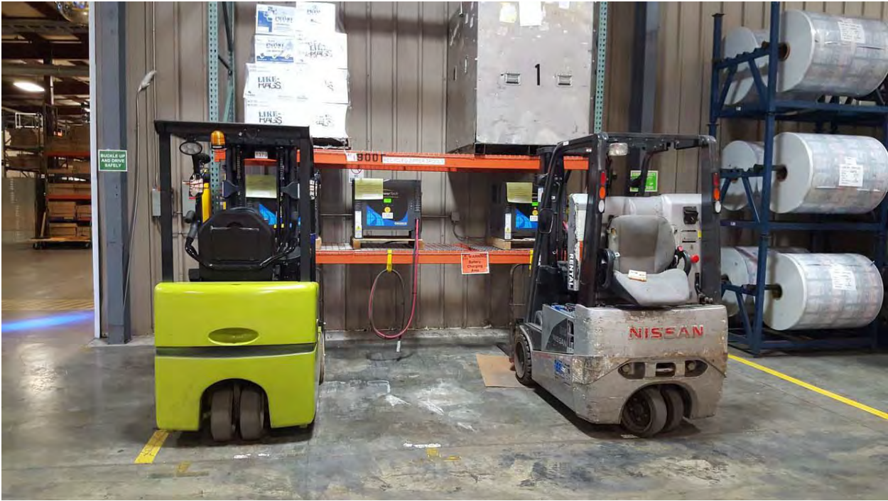
Battery Charging Station in the Warehouse
