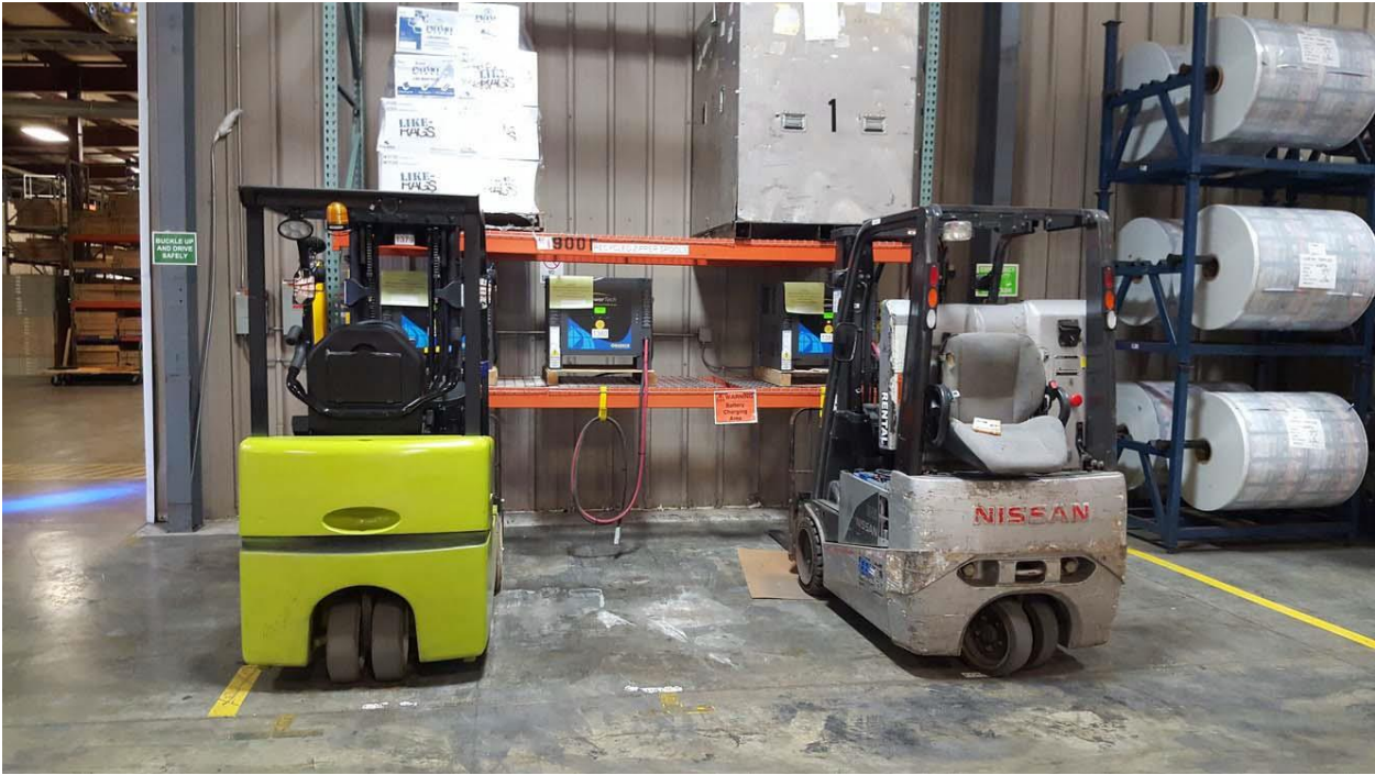
Battery Charging Station in the Warehouse
